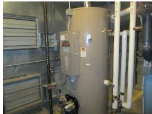
Lakeview ES DHW Heater
