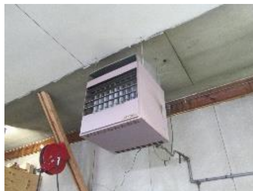
Bus Garage Unit Heater Bay 2
