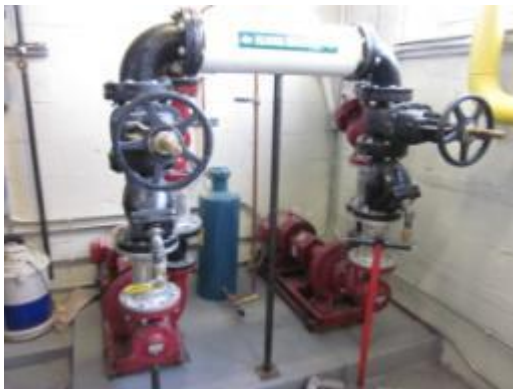
Lakeview ES Boiler Room Hot Water Pumps
