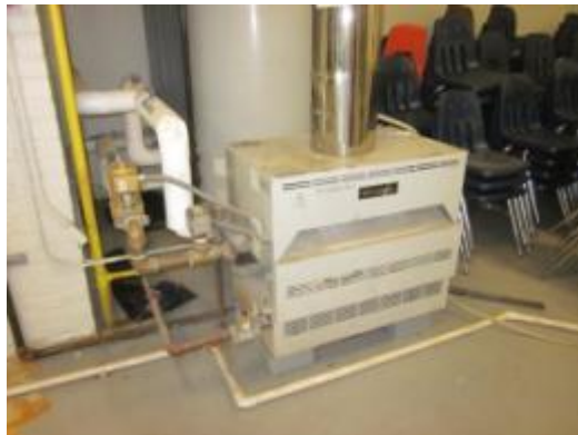
Valleyview Middle School DHW Heater
