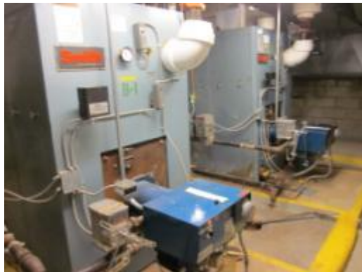
Lakeview Elementary School – Smith Boilers
