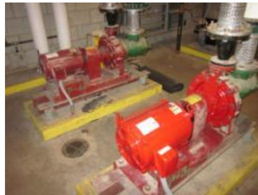
Lakeview ES Mezz. Mechanical Room Hot Water Pumps
