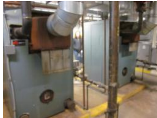
Lakeview Elementary School – Smith Boilers
